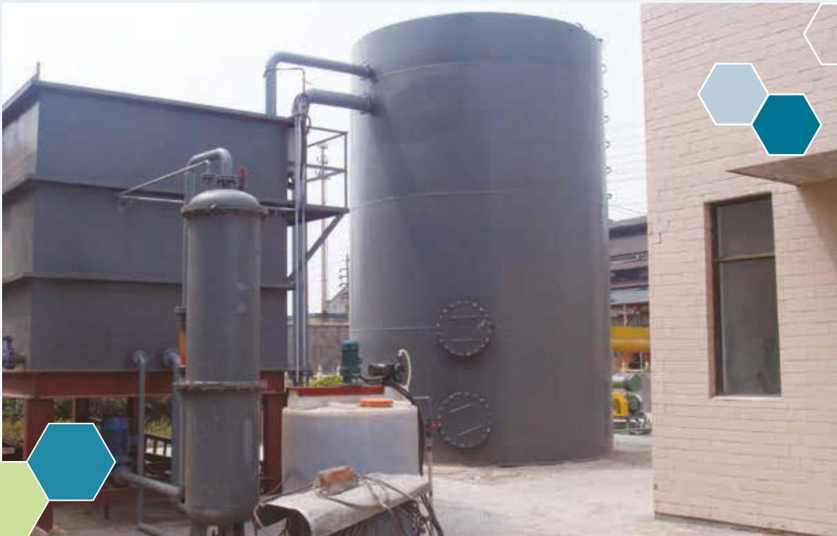
Wastewater treatment system
